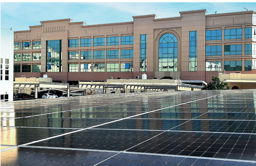
Mediclinic Solar Car Park Al Garhoud 410.43 kWp
