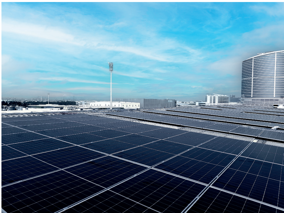
DHL Warehouses Dubai JAFZA 1.2 MWp
